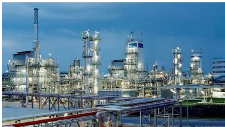
Figure 8.10 - Linde HyCO Plant. (Source: HyCO Plants|Linde Gas (linde-gas.com)
