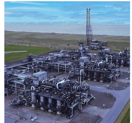
St. Fergus Gas Terminal, Peterhead Scotland
