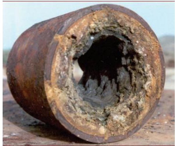
Figure 1: Mixed silica and sulphide scales in a reinjection pipe
